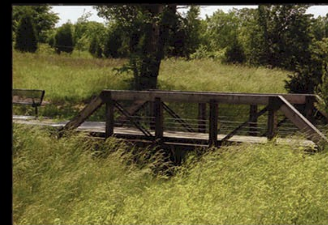
POINT OF INTEREST - bridge location - prefabricated bridge allows for minimal disturbance in PMJM habitat - potential bench and trash receptacle
